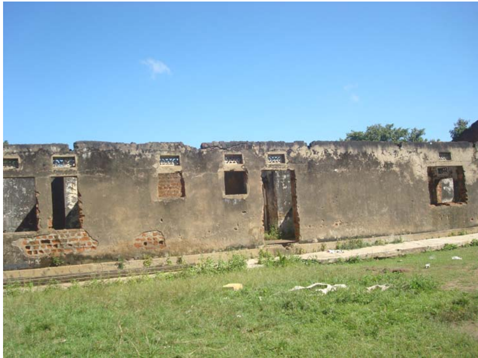
Plate 4.3: A house of a UNRF 1 ex-combatant that has not been reconstructed since the 1979 war in Yumbe district
