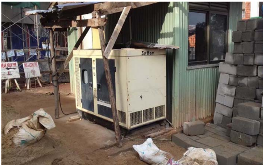
Figure 8: Stand-by Generator for Lighting and heavy duty machinery works in emergency need.
