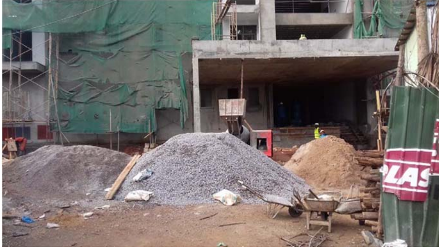
Figure 12: Concrete batch plant at site. In view is a small mixer machine
